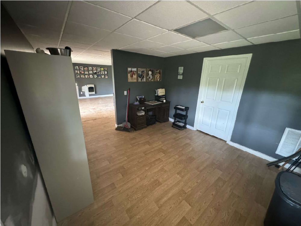
Indoor kennel room with example kennel set up. (Room is currently undergoing repairs from termite damage done during previous owners occupancy.)
