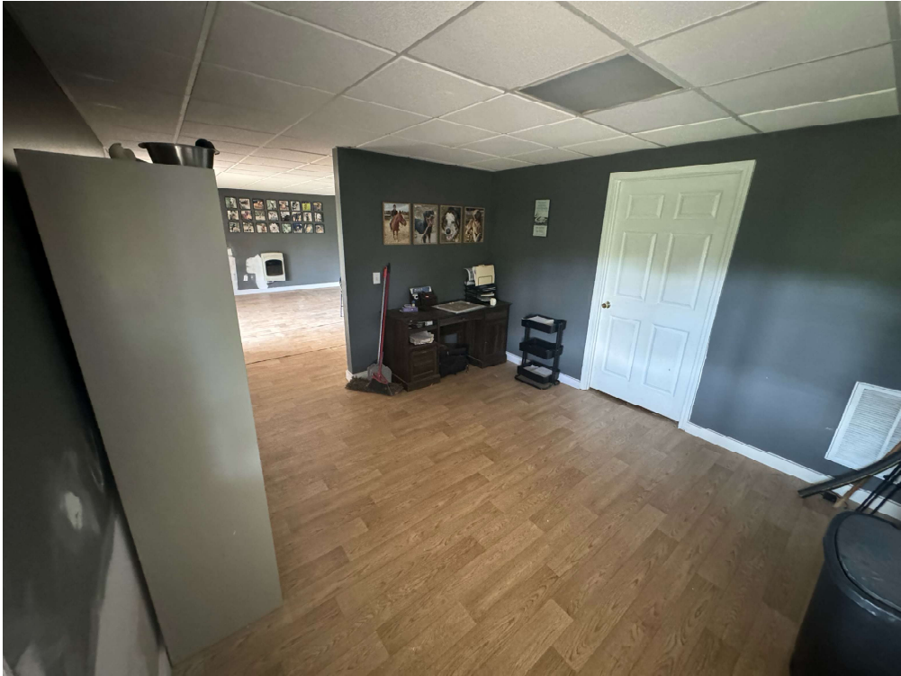
Indoor kennel room with example kennel set up. (Room is currently undergoing repairs from termite damage done during previous owners occupancy.)
