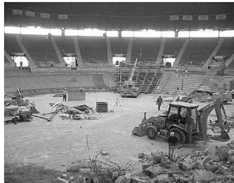
Construction crews spent over a year transforming the former Levitt Arena into Charles Koch Arena.
