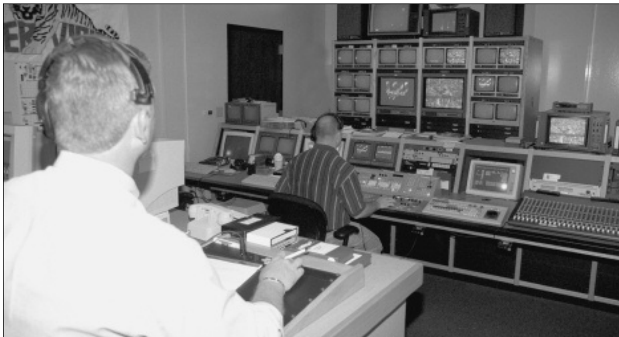
The Athletics Administration building houses a television control room that is used for video scoreboard broadcasts in Tiger Stadium and the Pete Maravich Assembly Center.
